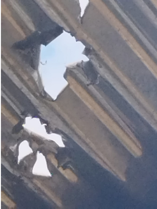
Bullet hole in roof of community home.
